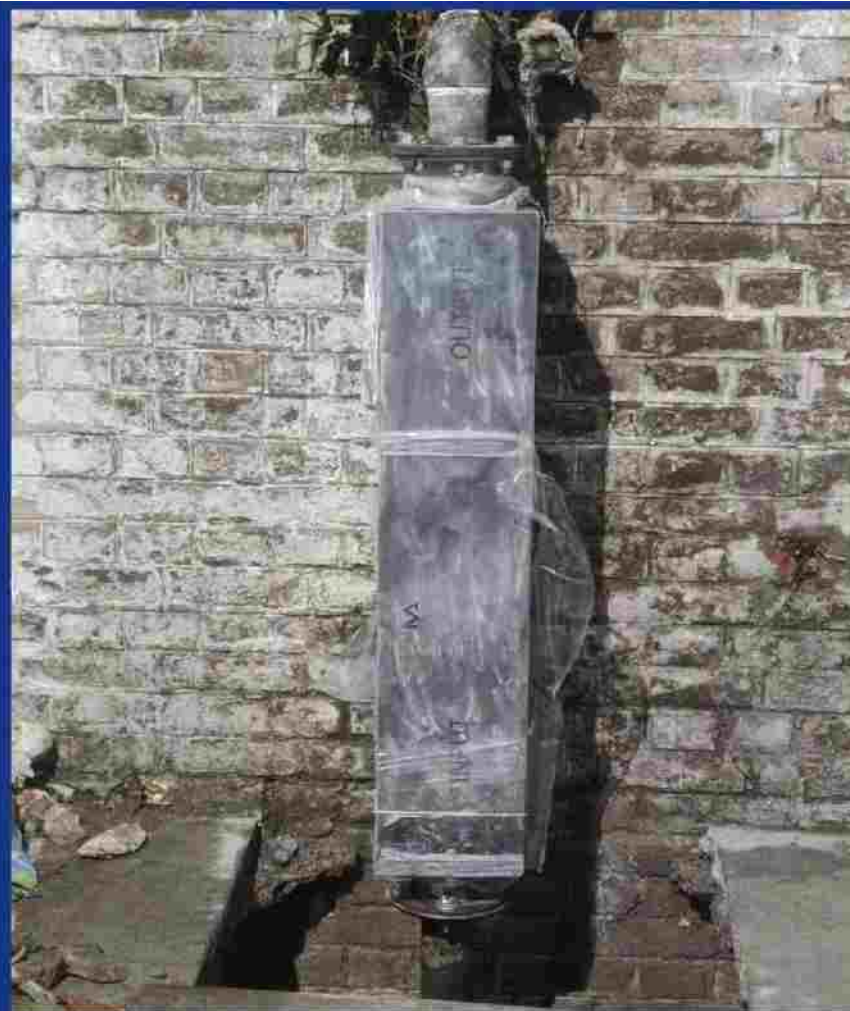
Installed at Shahdara Junction
